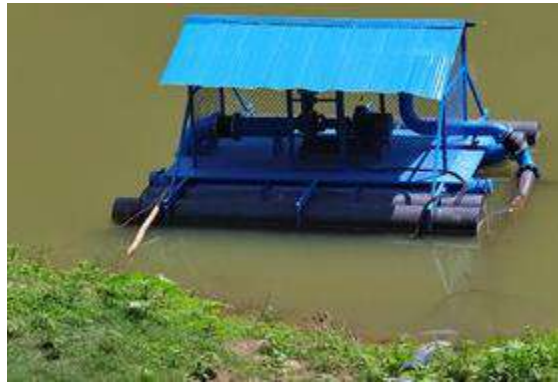
Figure 5.5:: Intake Pontoon Station
