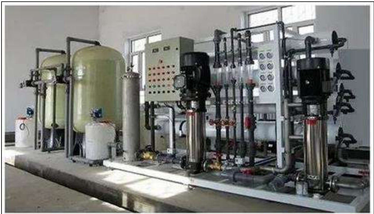
Figure 4.5: Reverse Osmosis Plant
