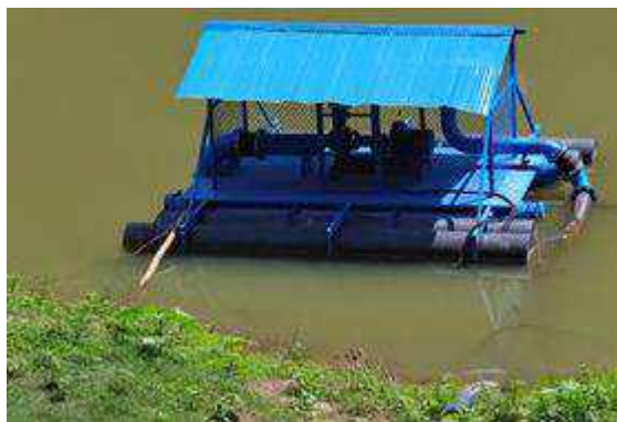
Figure 5.3: Intake Pontoon Station
