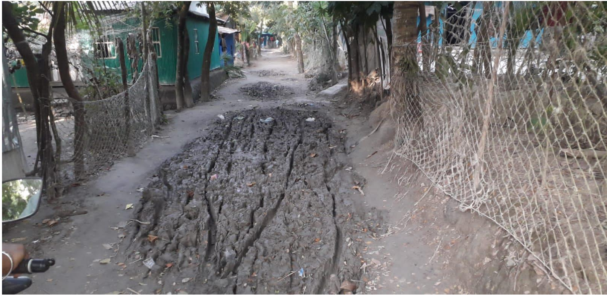
Figure 8: Condition of the visited road alignment at case study union
