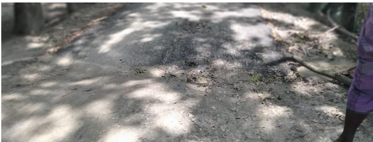
Figure 5: Condition of the visited road alignment at Case Study Union
