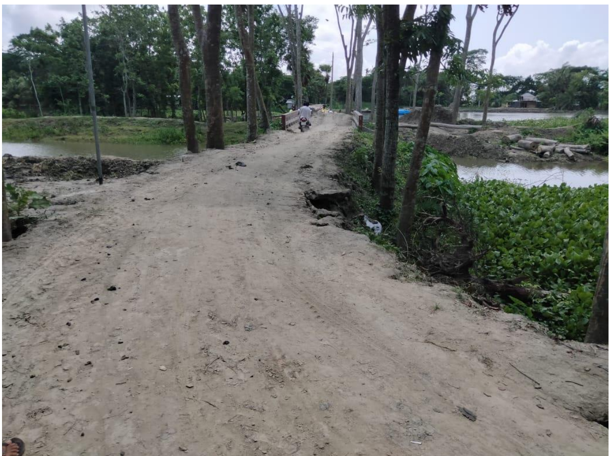
Figure 9: Condition of the visited road alignment at Case Study Union
