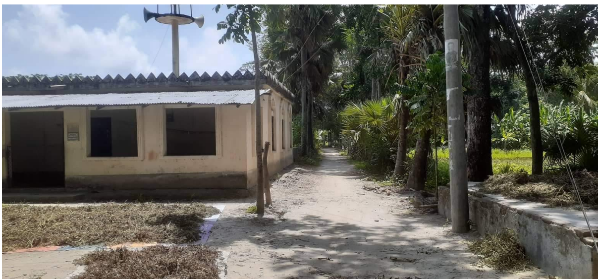
Figure 14: Condition of the visited road alignment at Case Study Union
