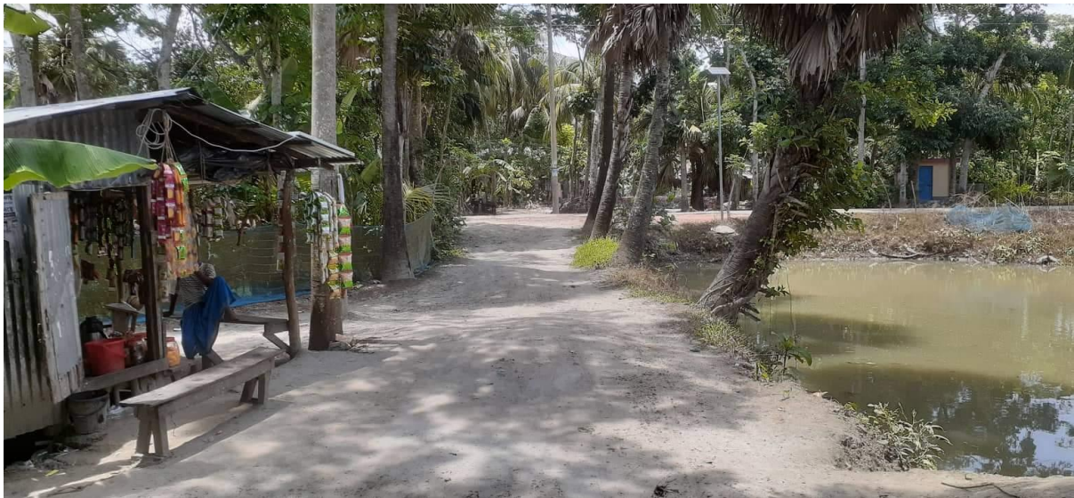
Figure 12: Condition of the visited road alignment at Case Study Union
