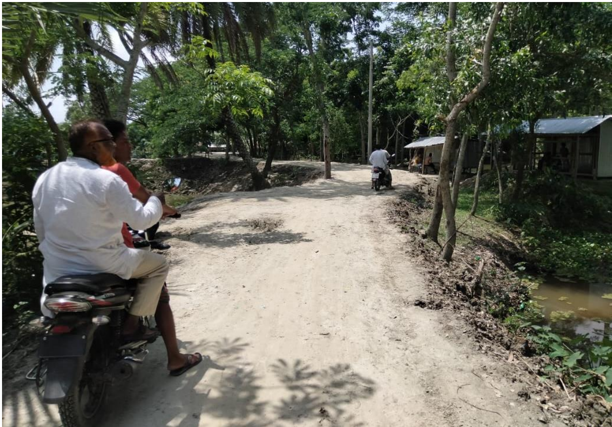
Figure 8: Condition of the visited road alignment at Case Study Union
