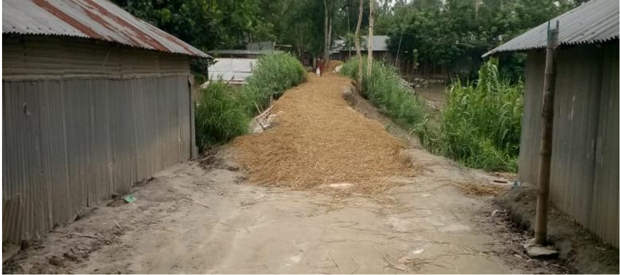
Figure 6: Condition of the visited road alignment at Case Study Union
