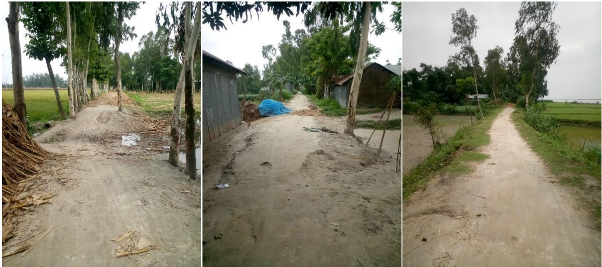
Figure 7: Condition of the visited road alignment at Case Study Union
