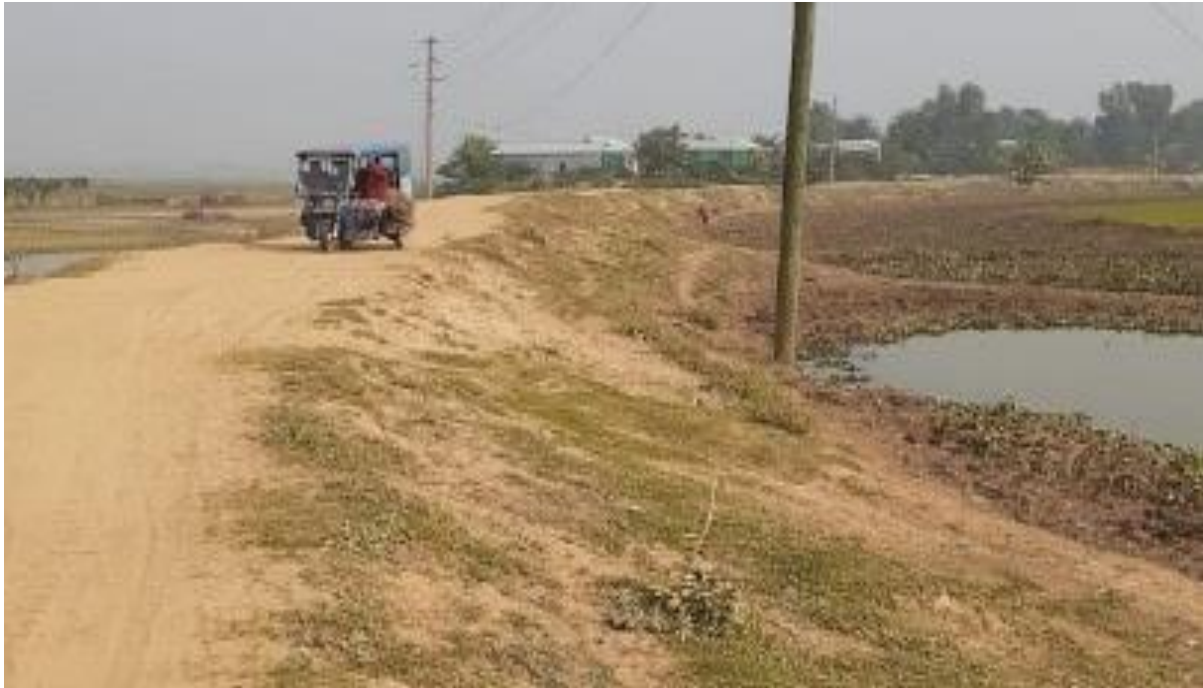
Figure 8: Condition of the visited road alignment at case study Union
