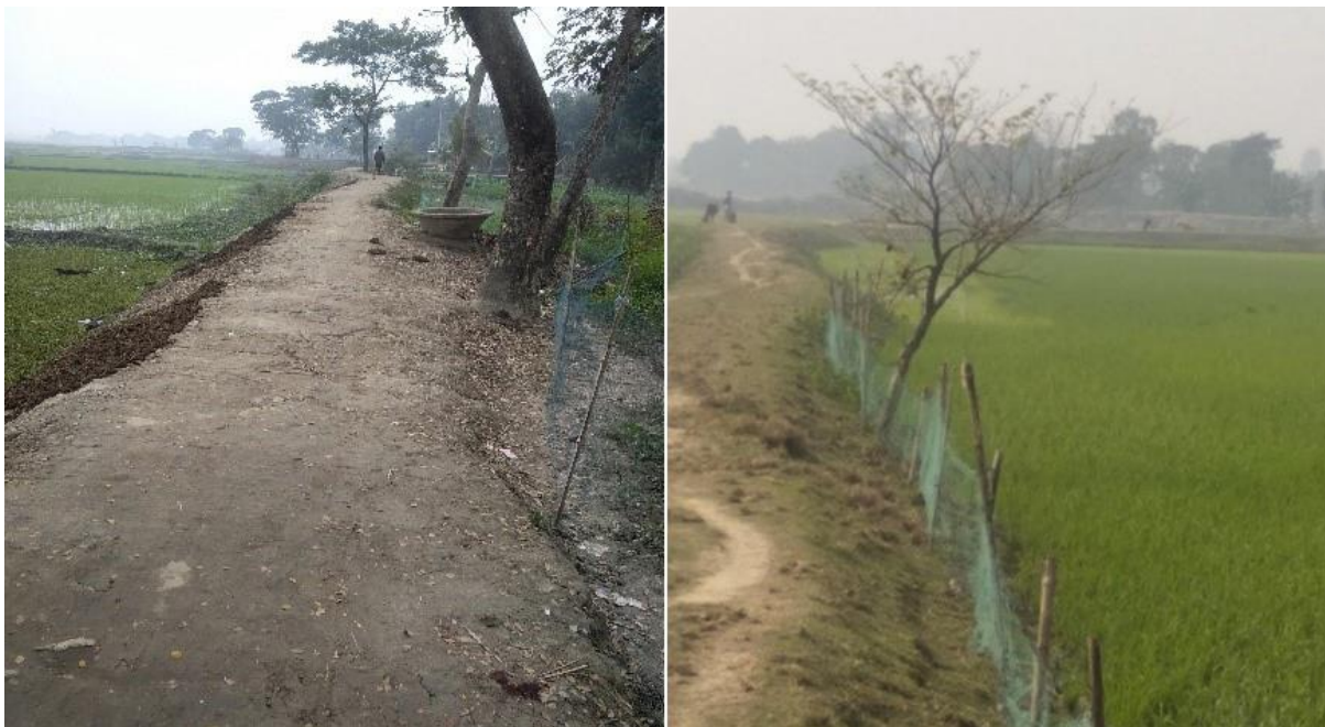
Figure 9: Condition of the visited road alignment at Badalpur Union
