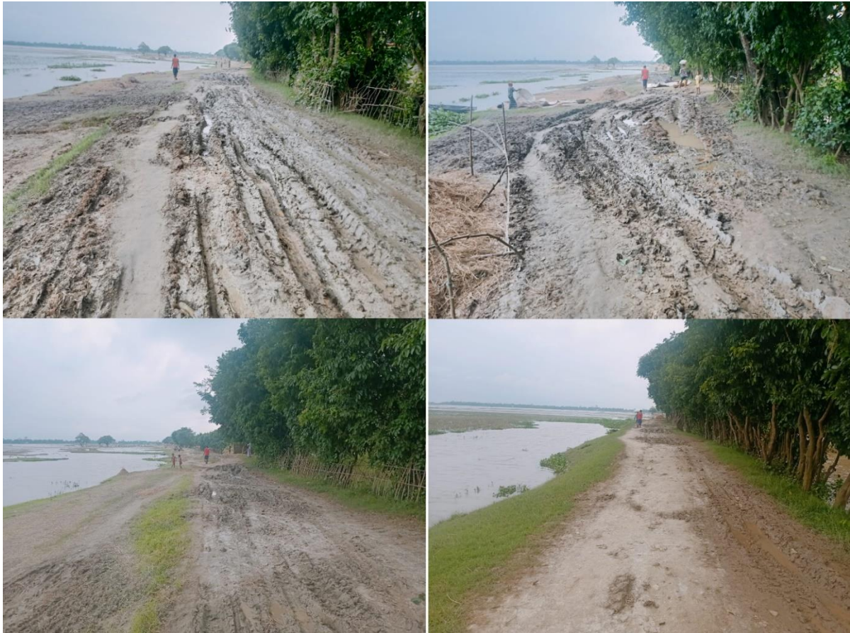
Figure 9: Condition of the visited road alignment (unpaved part 690933010)
