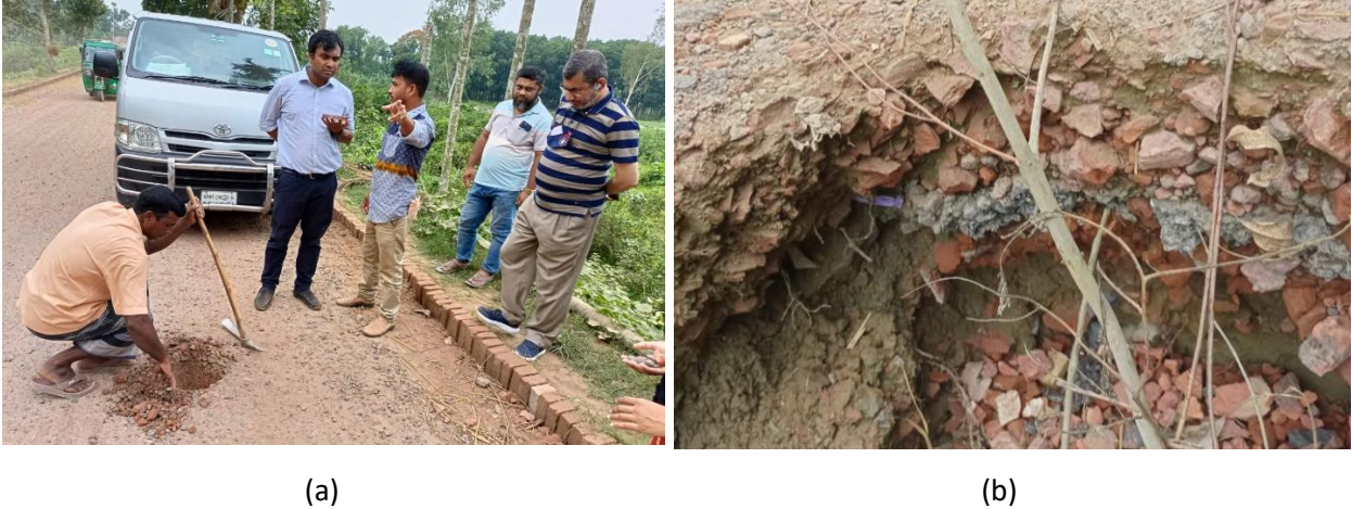
Figure 2: (a) Sample aggregate collection from widened road sub-base. (b) Typical section of widened road (up to sub-base)
