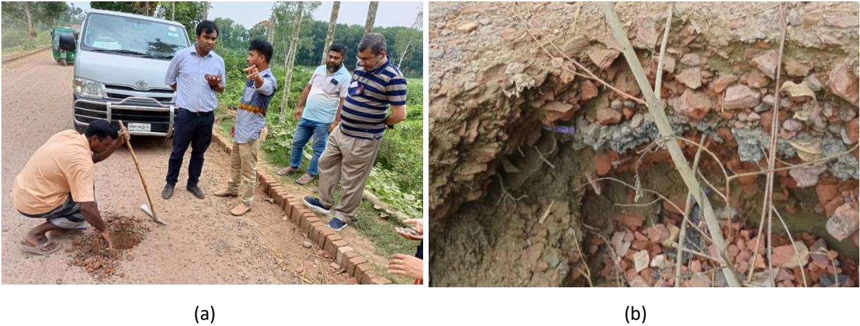
Figure 2: (a) Sample aggregate collection from widened road sub-base. (b) Typical section of widened road (up to sub-base)
