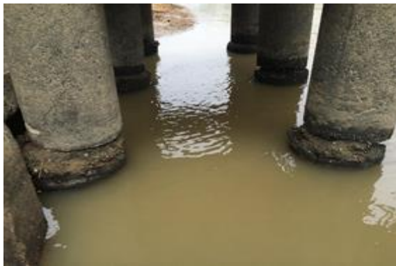
SB3. Lack of continuity
