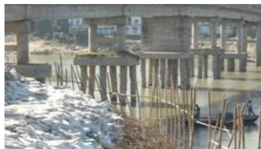
SD4. Scour and erosion
