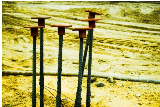
Rebars safety protrudes (caps)
