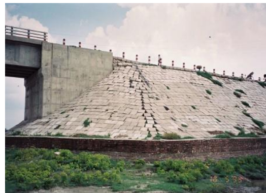
EM2. Excessive deformations
