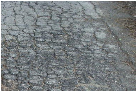
FP1. Surface cracking (alligator cracking)
