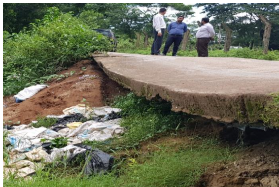
EM1. Scour and wash-out
