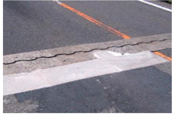
SB2. Movement joints malfunctioning
