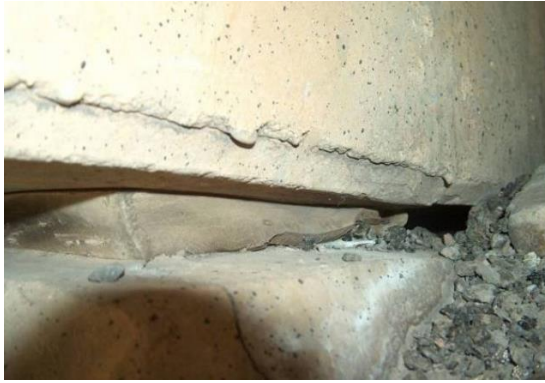
SB1. Bearing Malfunctioning
