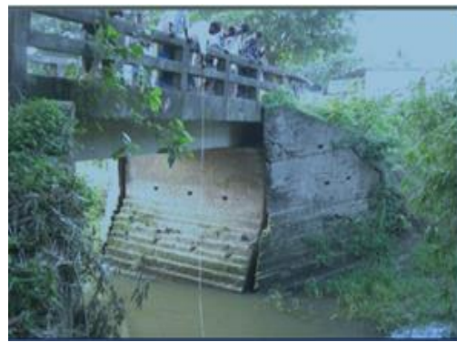
Bridge Failure: Leaning and Settlements
