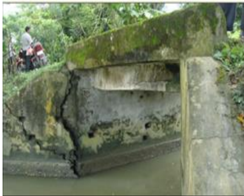
Bridge Failure: Settlements
