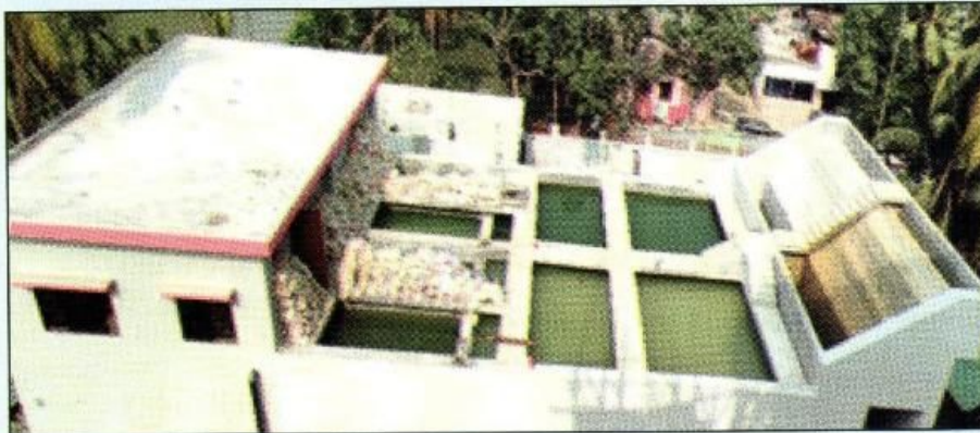
Groundwater treatment plant under construction in Laxmipur Municipality with the support of UGIIP-3 project
