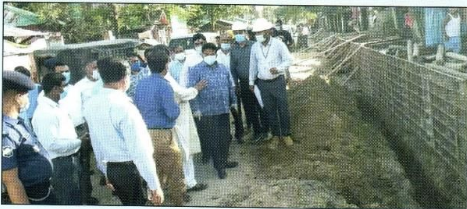
Senior Secretary of Local Government Division Helal Uddin Ahmed visiting Cox's Bazar municipality infrastructure development works on 2 October 2020
